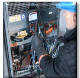
Power Quality Testing
